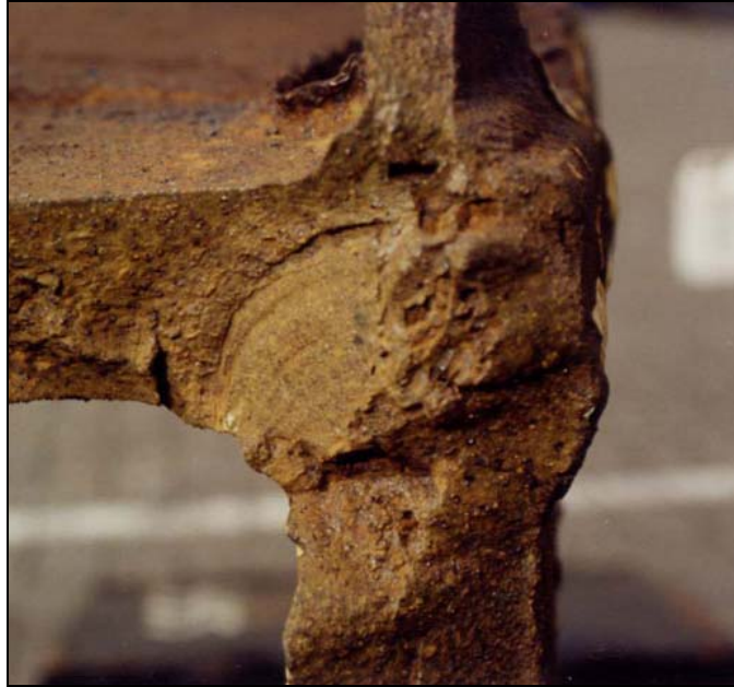
Figure 8. Excessive Weld Material, Port Side Joint
